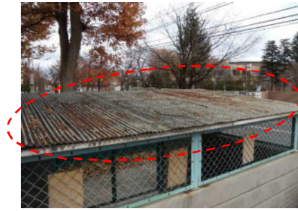
●ゴミ置場屋根の錆
